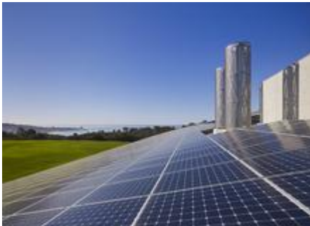
Photovoltaic panels help power the building. - Photo Credit: © Nick Merrick
