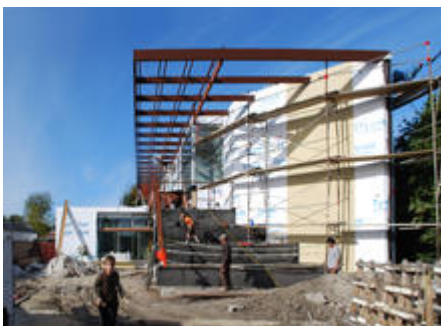
Construction view showing large overhang that shades the home - Photo Credit: Lawrence Scarpa
