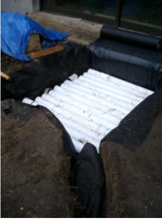
Installing the low tech stormwater system with stacked perforated pipe and gravel - Photo Credit: Brooks Scarpa
