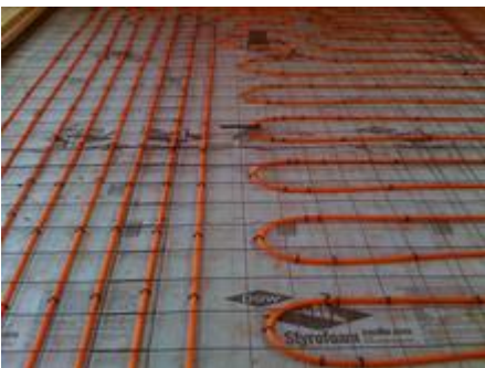
Thermally broken radiant slab ready for 50% flyash topping slab - Photo Credit: Lawrence Scarpa
