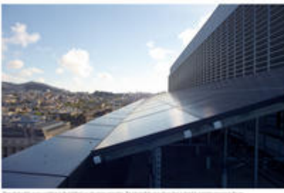
Photovoltaic arrays - Photo Credit: Photographs ©2012 Bruce Damonte. All rights reserved.
